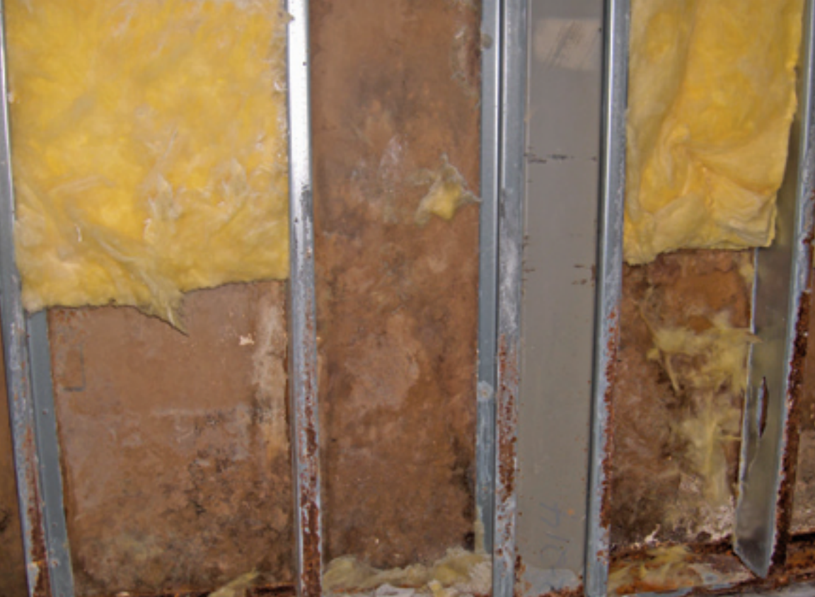
Water damage at Expertint photo provided by Expertint
