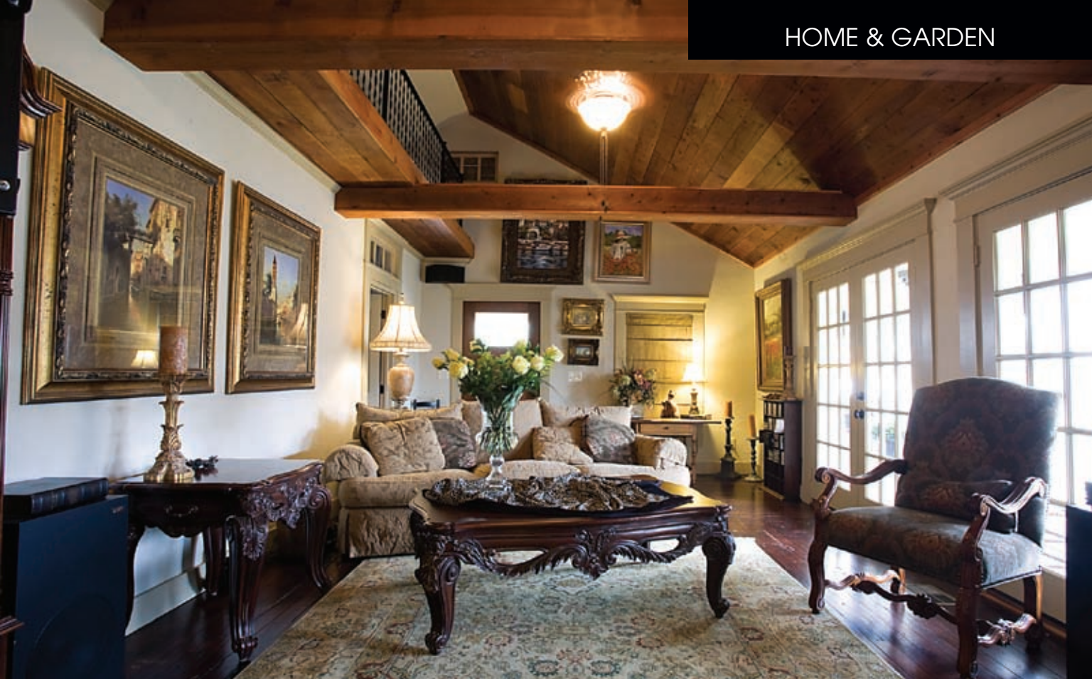
The original wood floors were removed, taken outside, cleaned up and reinstalled. The Messinas raised the roof for a more open feel.
