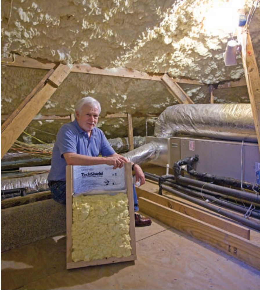
Jim Sargent found controlling the attic environment enables greater energy efficiency. photo by Chris Frütche
