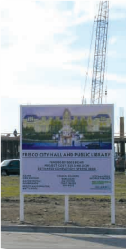
City Hall construction (top), the construction of IKEA from the Dallas North Tollway, (bottom) photos by Chris Johnson
